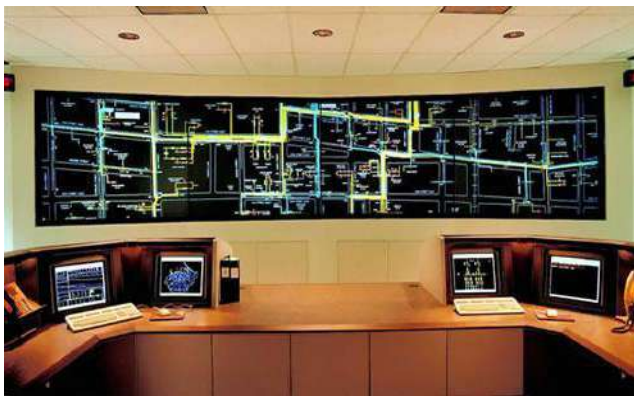
Fig. 3. Central Control Room
